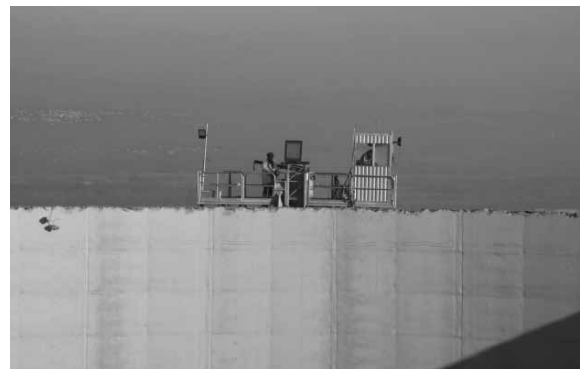
Figure 2: Conventional operation of the excavator with a handheld remote control from a platform on top of the cooling tower.
